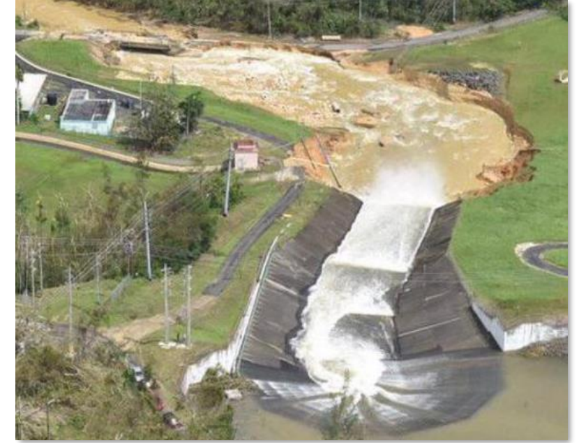
Guajataca Dam spillway failure
