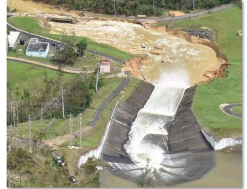
Guajataca Dam spillway failure
